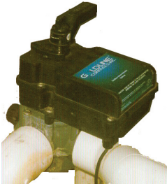
Automatic valve control
